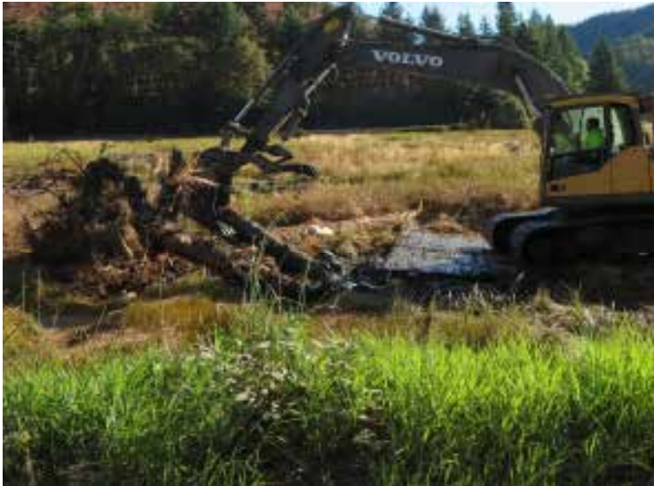
Figure 3. Log placement creates large wood fish cover, pool scour, and elevation diversity in a tidal marsh. Photo courtesy of Fran Recht, PSMFC
