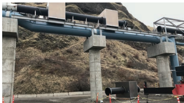
Installation of three antenna systems on new full flow bypass at Lower Granite Dam. Photo courtesy of Scott Livingston, PSMFC
