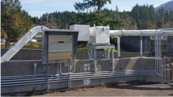
Additional antennas added for Lamprey Bypass System at Bradford Island Ladder of Bonneville Dam. Photo courtesy of Scott Livingston, PSMFC
